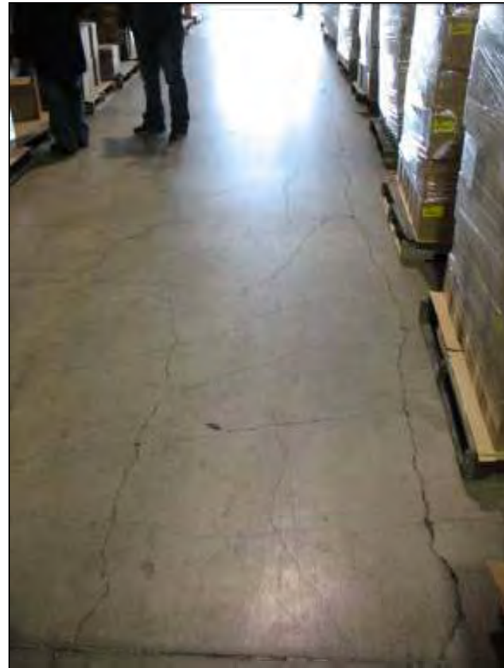
Random crack pattern
