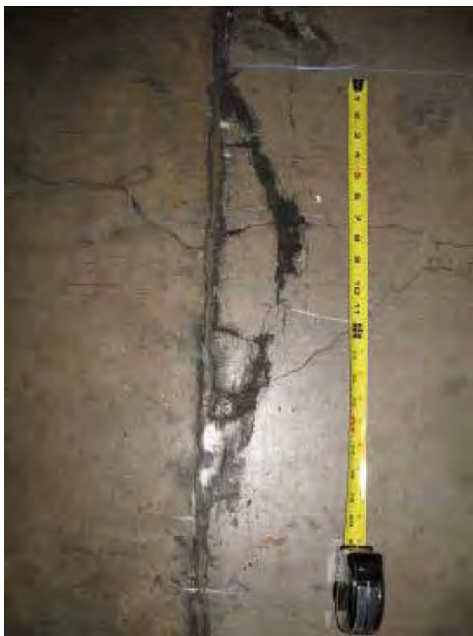
Spall and cracks at control joint
