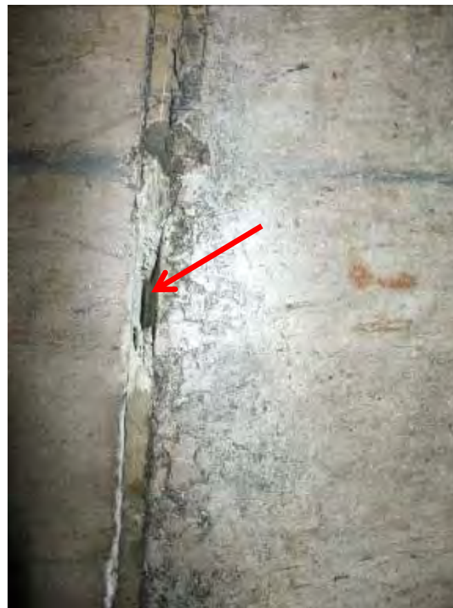
Missing control joint material (arrow)
