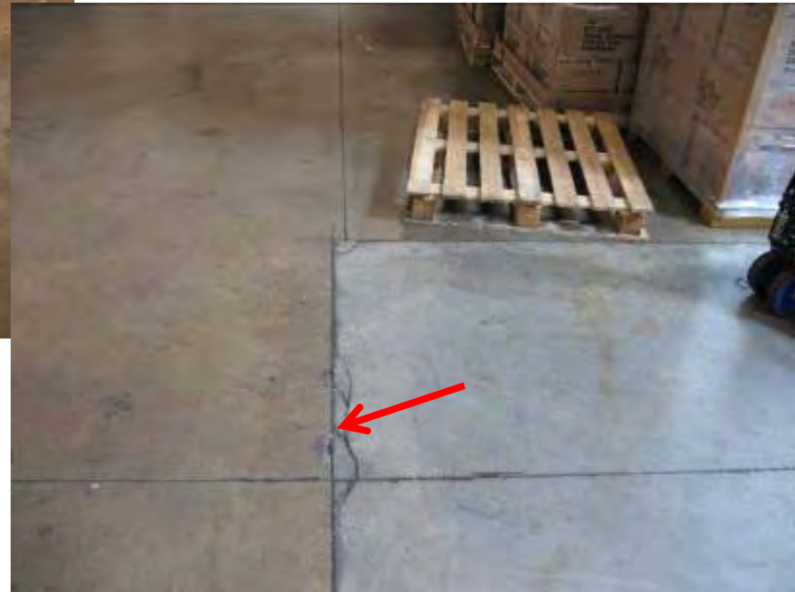
Spall at edge of new concrete placed at equipment at overhead door (see arrow)
