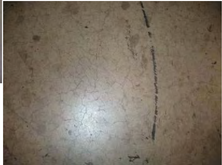
Surface crazing cracking
