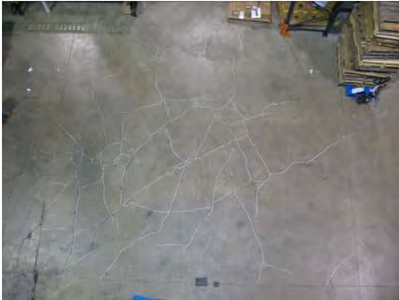
View of a crack pattern thought to be from a crane load stabilization point
