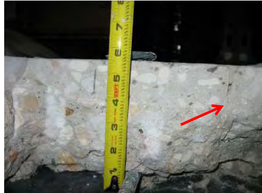
Rebar located at the bottom of the slab. Note no cracking propagating from bottom of the control joint. (arrow).
