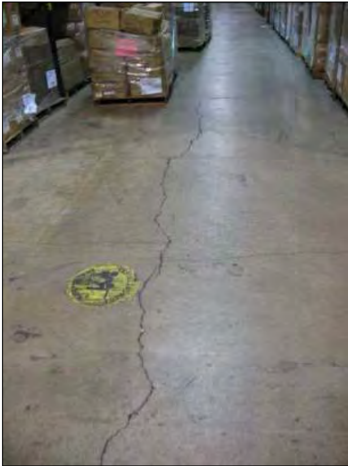
Typical cracks located roughly in the middle of an aisle
