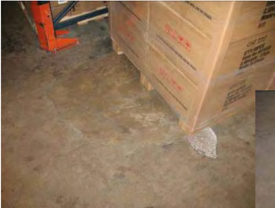
Surface spall next to a pallet
