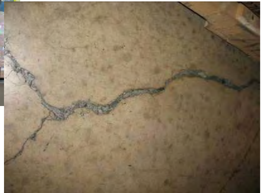
Crack previously repaired with epoxy injection Al Bustamante, Wiss, Janney, Elstner Associates, Inc.
